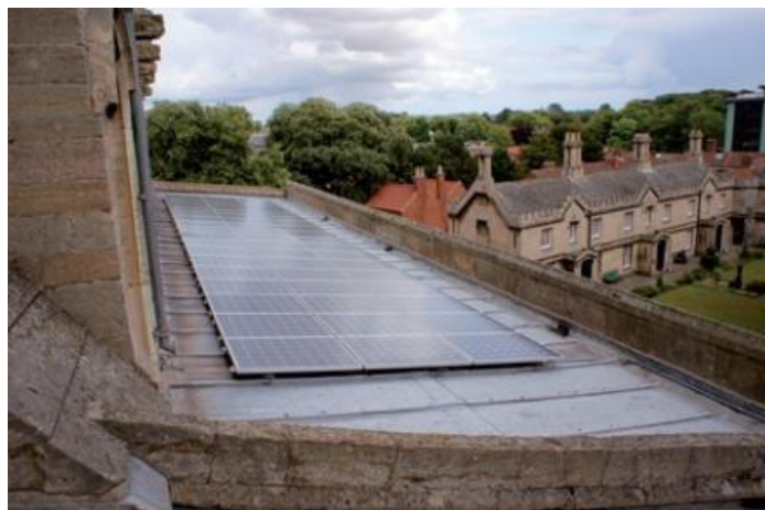
A typical PV arrangement on a church roof
